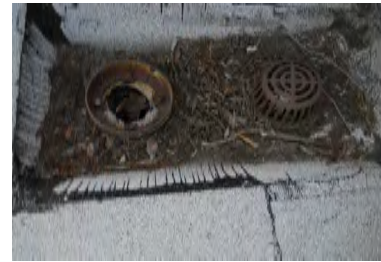
Typical Deficiency - Observed debris at field of roofing. Recommend clearing debris from all gutters, drains, waterways, and field of roof to promote positive drainage.
