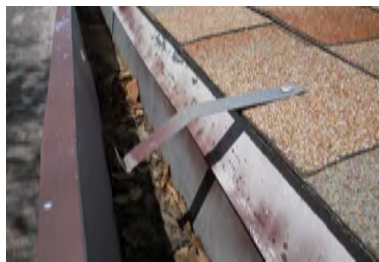
Typical Deficiency - Gutter brackets have been face fastened through asphalt shingle. Recommend removal and repositioning bracket. Repair asphalt shingles as needed.
