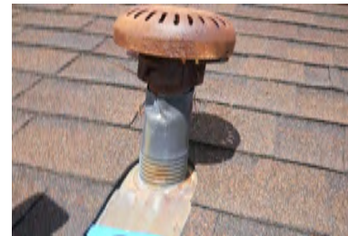
Typical Deficiency - Pipe jacks are missing band clamps and sealant. Recommend installing stainless steel band clamps, apply sealant, and install storm collar.
