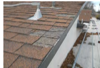
Typical Deficiency - Shingles are missing. Recommend replacing as needed.
