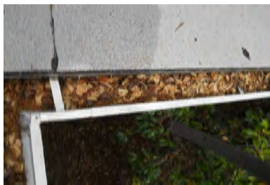
Typical Deficiency - Gutters are full of debris. Recommend clearing debris from all gutters, drains, waterways, and field of roof to promote positive drainage.
