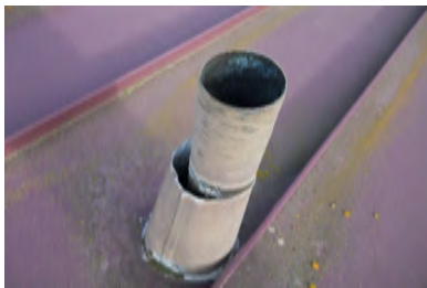
Typical Deficiency - Pipe jacks are missing sealant. Recommend application of flexible flashing self-adhered tape and or sealant, and install storm collar.
