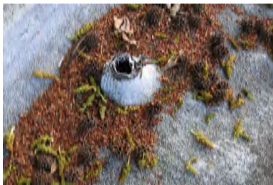
Typical Deficiency - Pipe jack at through roof penetration is damaged. Recommend repairing as needed.
