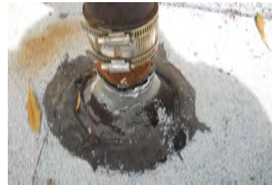
Typical Deficiency - Through roof penetrations do not appear to have proper low slope roof jack. Recommend installing proper roof jack and storm collar.
