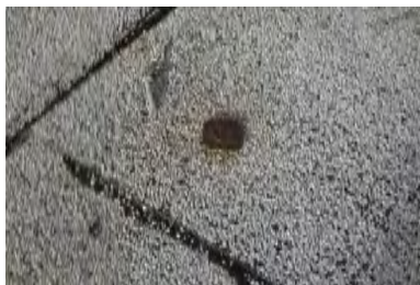
Typical Deficiency - Observed fastener penetrating through finished built-up roofing. Recommend removal and patch.
