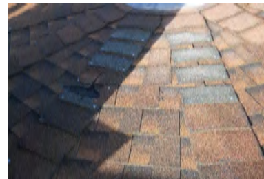
Typical Deficiency - Hip and ridge shingles are missing. Recommend replacing as needed.
