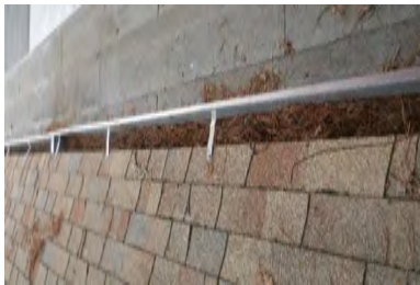
Typical Deficiency - Gutter brackets have been face fastened through asphalt shingle. Recommend removal and repositioning bracket. Repair asphalt shingles as needed. Typical Deficiency - Gutters are full of debris. Recommend clearing debris from all gutters, drains, waterways, and field of roof to promote positive drainage.
