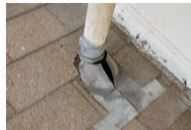
Typical Deficiency - Pipe jack is open. Recommend removal and replacement and installation of storm collar.
