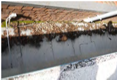
Typical Deficiency - Observed accumulation of debris at field of roof. Recommend clearing debris from all gutters, drains, waterways, and field of roof to promote positive drainage.
