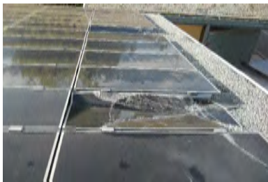
Typical Deficiency - Damaged solar panels. Recommend further investigation and repair by licensed solar contractor.
