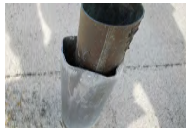
Typical Deficiency - Pipe jacks are missing sealant. Recommend application of flexible flashing self-adhered tape and or sealant, and install storm collar.
