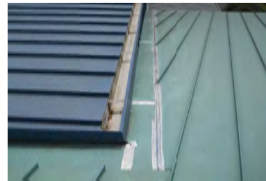
Typical Deficiency - Roof transition/ cricket has been temporarily sealed. Recommend removal of all temporary repairs and installation of as needed permanent repairs.
