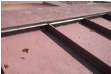
Typical Deficiency - Ridge closure pieces have buckled. Recommend removal and reinstallation as needed.
