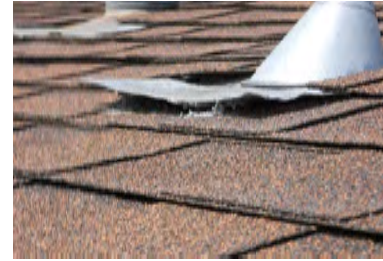
Typical Deficiency - Pipe jacks are damaged. Recommend installing new GSM roof jack and storm collar.
