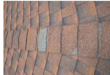
Typical Deficiency - Hip and ridge shingles are missing. Recommend replacing as needed.
