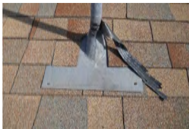
Typical Deficiency - Sealant at steep slope roof jack needs to be replaced. Recommend re-seal and install storm collar.
