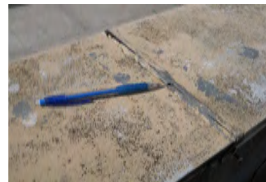
Typical Deficiency - Sealant at coping seams has begun to fail. Recommend removal and replacement of sealant as needed.
