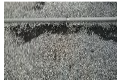
Typical Deficiency - Areas of displaced gravel. Recommend re-distributing and adhering gravel over bare areas to protect underlying membrane from exposure to UV .
