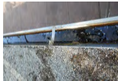
Typical Deficiency - Gutters are full of debris. Recommend clearing debris from all gutters, drains, waterways, and field of roof to promote positive drainage.
