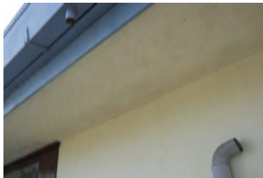
Typical Deficiency - Missing leader pipe. Recommend installation of leader pipe to divert water to lower roof.
