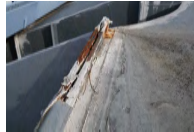
Typical Deficiency - Mechanical duct work seams damaged and deteriorated. Recommend replacement of damaged duct by licensed mechanical contractor and coating with acceptable silicone or acrylic coating.
