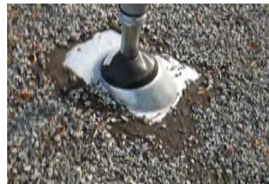
Typical Deficiency - Through roof penetrations do not appear to have proper roof jack. Recommend installing proper roof jack and storm collar.
