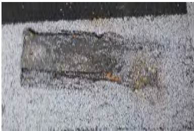
Typical Deficiency - Mineral surfaced cap sheet is damaged from previous sleeper block that has been removed. Recommend repairing as needed.
