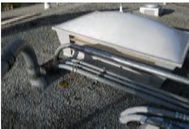
Leak Reported Below. Recommend further review and assessment.
