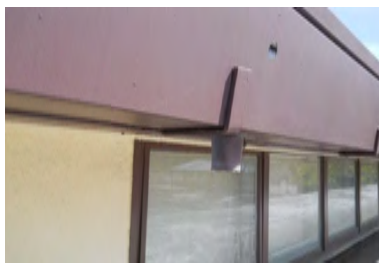
Typical Deficiency - Missing leader pipe. Recommend installation of leader pipe to divert water to lower roof.
