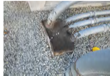
Typical Deficiency - Pitch pocket sealants have dried out and pulled away from flashing. Recommend topping off pitch pocket with compatible sealer or modified mastic and application of acrylic or silicone coating to preserve and maintain repair.
