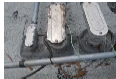
Typical Deficiency - LB electrical penetrations have not been flashed properly. Recommend installing galvanized pitch pocket with cover.
