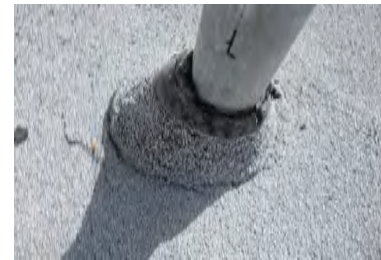
Typical Deficiency - Through roof penetration is open. Recommend resealing and installing storm collar.
