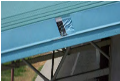
Typical Deficiency - Metal fascia detail is incomplete. Recommend repairing as necessary to provide a water tight application.
