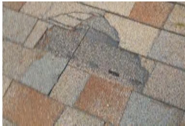
Typical Deficiency - Asphalt shingles are damaged and missing. Recommend replacing as needed.
