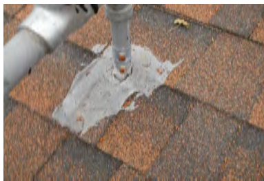
Typical Deficiency - Through roof penetrations do not appear to have proper roof jack. Recommend installing proper roof jack and storm collar.
