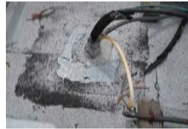
Typical Deficiency - Condenser line sets and electrical have not been flashed properly. Recommend installing galvanized pitch pocket with cover.
