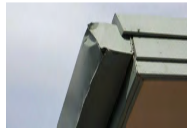
Typical Deficiency - Corner of gutter is damaged. Recommend repair and seal as needed.
