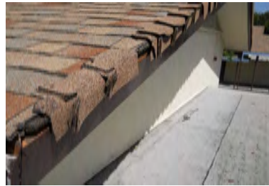
Typical Deficiency - Hip and ridge shingles are damaged and missing. Recommend replacing as needed.
