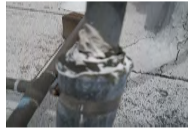
Typical Deficiency - Sealants at pipe jacks have dried up and pulled away. Recommend removal/ replacement of sealant, and install storm collar.
