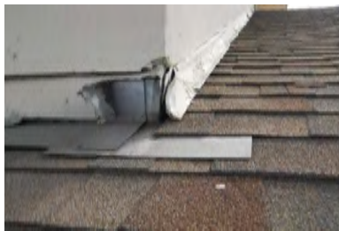
Typical Deficiency - Roof to wall counter flashing is open. Recommend removal and replacement as necessary to achieve water tight application.
